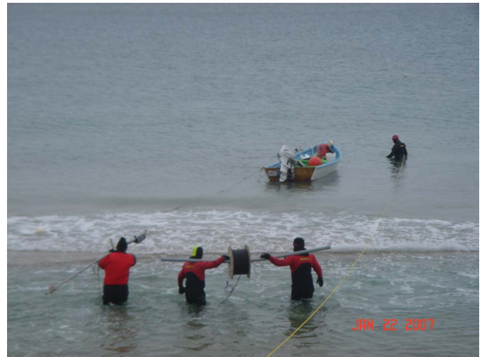
Fig. 6 Deployment of cable to the installation site 250 meters offshore at Madaket on a calm day. Electrical cable is tie wrapped to 3/8" galvanized chain every 1.5 m.
